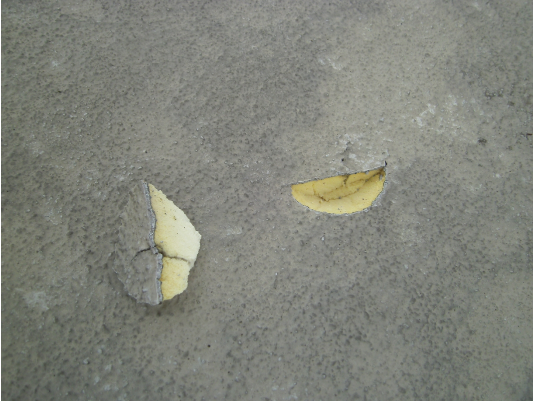
Photo 3 This crack extends 3/4 inch into the foam and showing the hail damage is more severe
