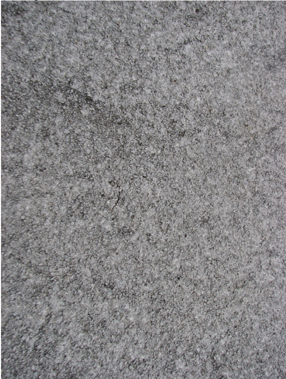
Photos 4 & 5 Granules can help reduce hail damage, but can also hide cracks unless investigated more closely
