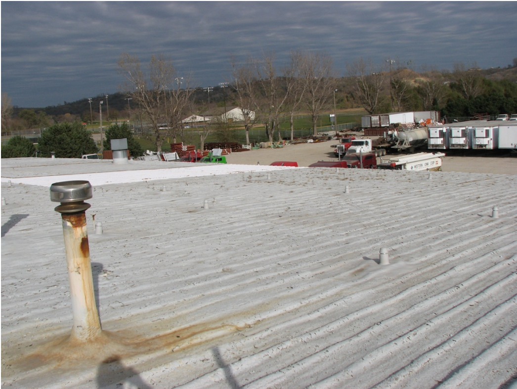
Photo 8 If you observe plants growing in the roof, it is too late to perform repairs in that section
