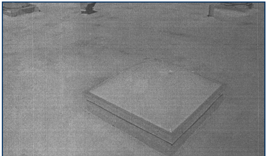
The skylight has been damaged by hail, but the SPF roof exhibits no visible signs of damage.
