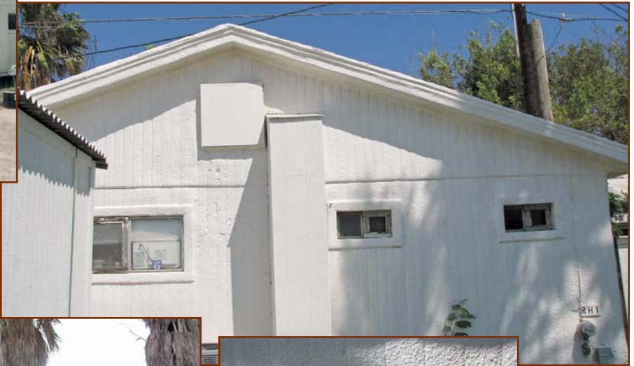
Figure 14 – Same building after Hurricane Dolly in 2009.
