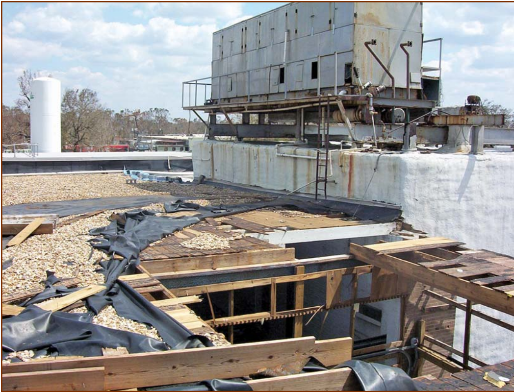
Figure 9 – Internal pressurization during Hurricane Katrina destroyed a tongue-and-groove wood deck at this ice plant.
